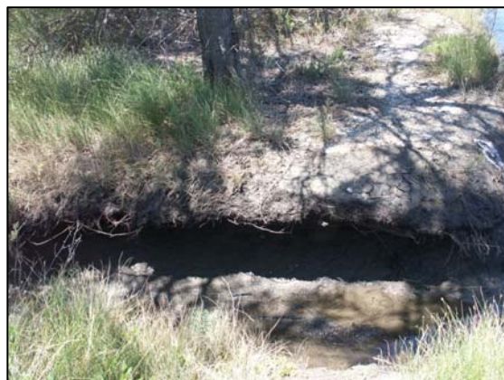
Erosion along drainage lines at Maylands Foreshore – City of Bayswater. Severe undercutting can be seen below the root zone (photo provided by NMCG).
