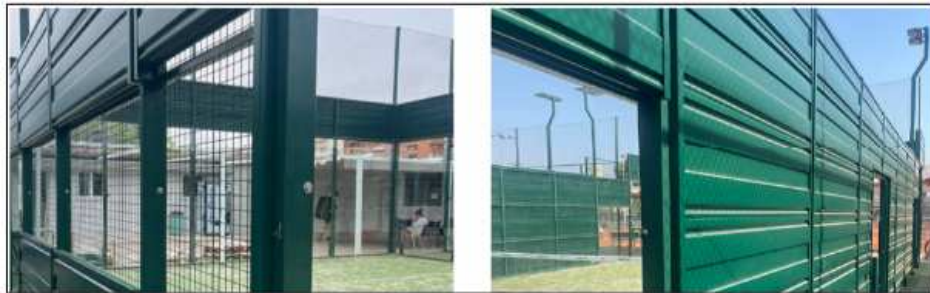
FIGURE G2 – PHOTO OF A PADEL COURT FITTED WITH THE ACOUSTIC PANELS
