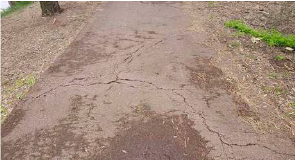
Paths in poor condition with uneven surface from cracking.
