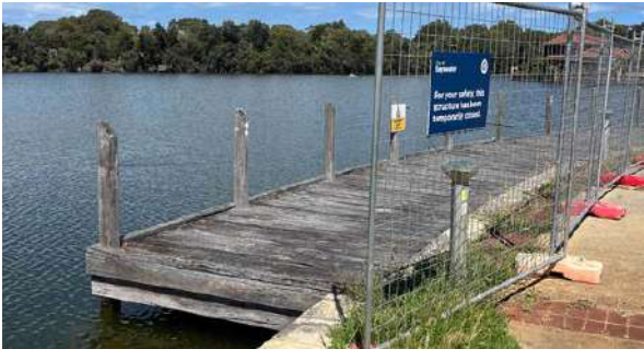
Boardwalk closed off for safety concerns.
