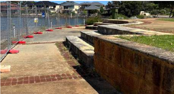
Terraced seating in degraded condition, safety concern from wall height.
