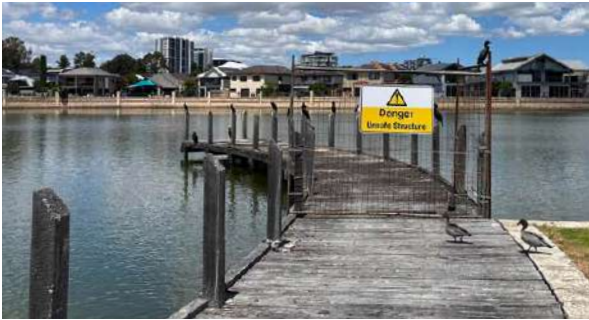
Boardwalk deteriorated, access closed from safety concerns.
