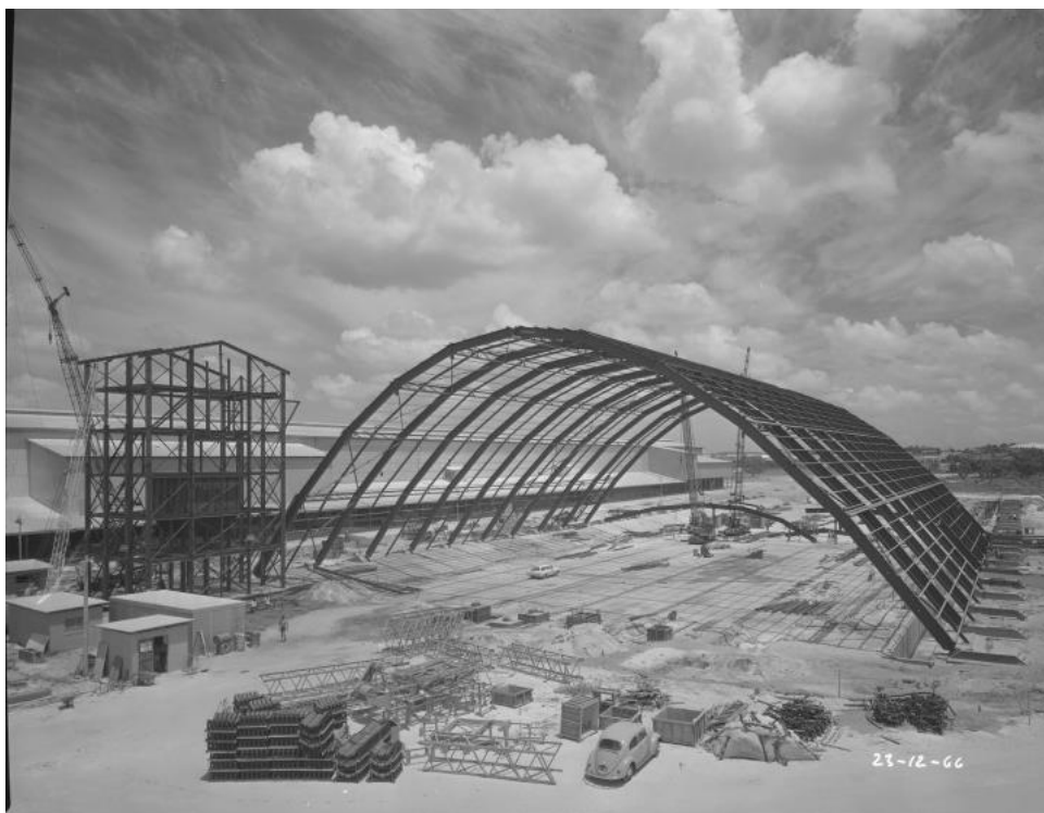
FIGURE 42 CONSTRUCTION OF A NEW SUPERPHOSPHATE DESPATCH PLANT AT CRESCO FERTILIZER FACTORY, 1966 Courtesy SLWA online image b3597941_7
